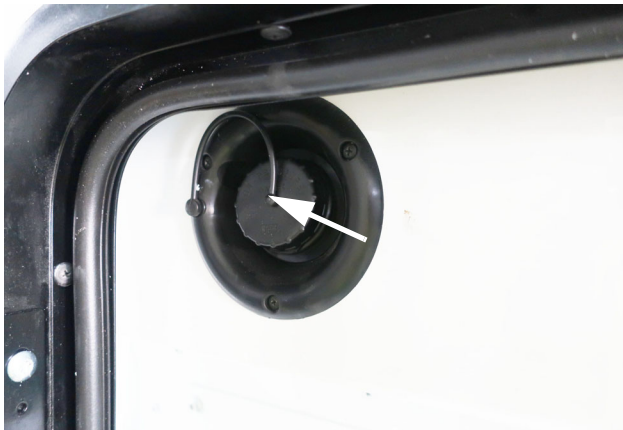
Water Tank Gravity Fill (Located in the Water Service Center) -Typical View
