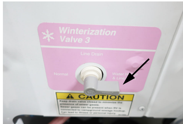
Winterization Valve 3 (Turn it to the Water Heater and Line Drain position). -Typical View
