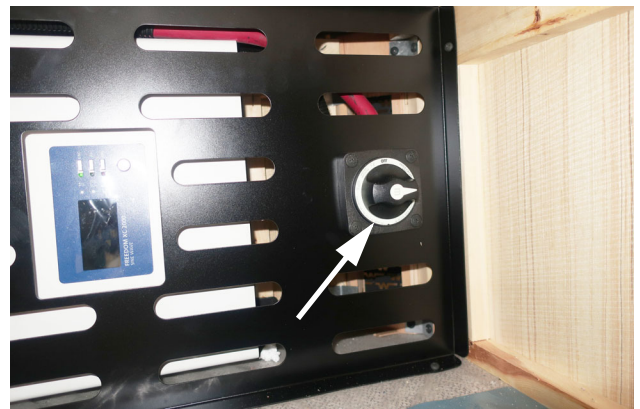
Inverter/charger disconnect switch. (Located inside the passenger's side compartment door next to the inverter). -Typical View
