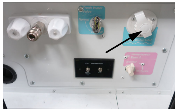
City Water Inlet (Located behind the drivers side Water Service Center door) -Typical View
