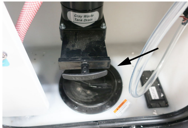
Sewage Drain Outlet with drain valve (Located inside the Water Service Center on the drivers side pull valve outward to open) - Typical View
