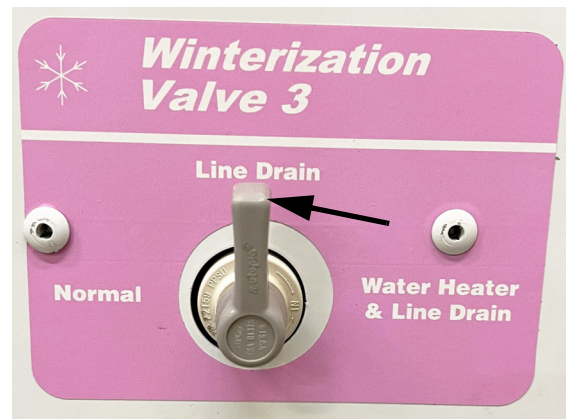
Winterization Valve 3 turned to the “Line Drain” position. -Typical View
